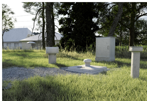
Installation d'une station Wilo-EMUport CORE.
